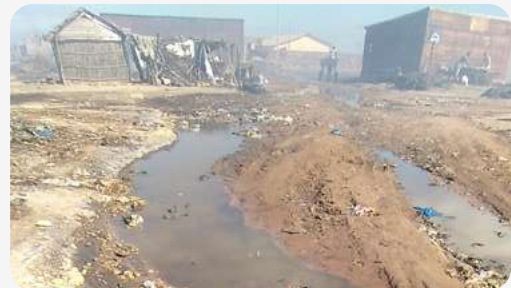
FIGURE 14: Water discharge allegedly coming from the nearby Omega Fishing SA FMFO factory in Joal Fadiouth, Senegal
